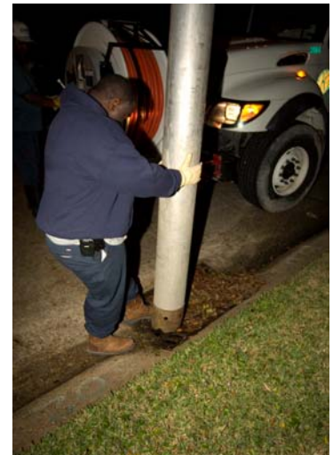
Kenner worker pulls debris from street drain in 3600 block of Tulane Drive.
